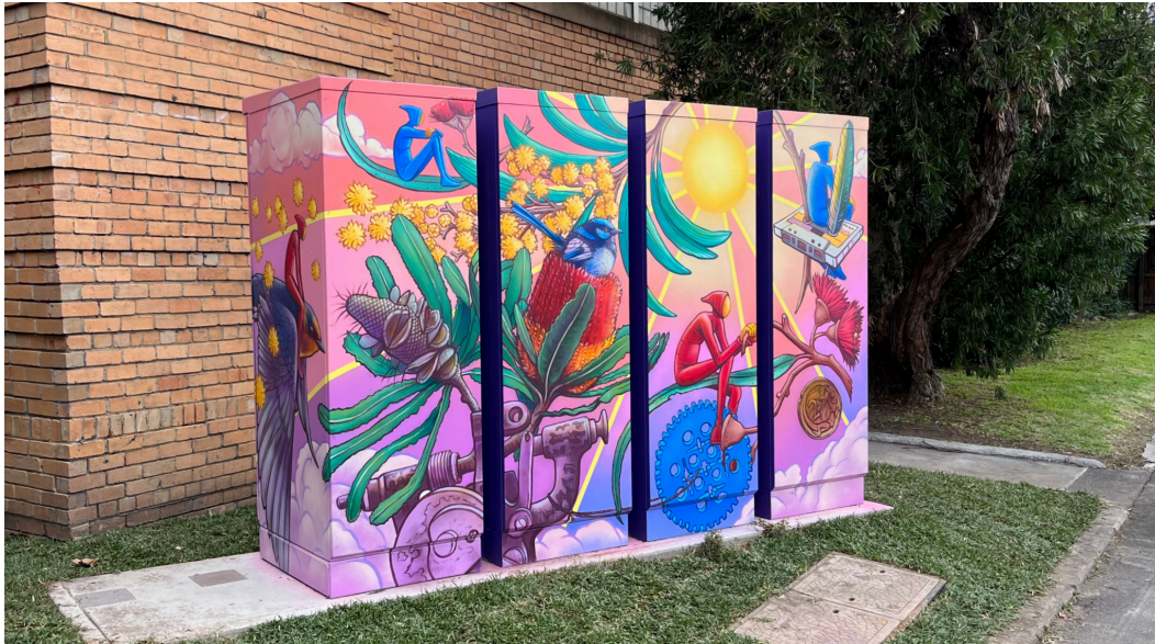
Figure 3. A 110 kW community battery in Melbourne, Australia, approximately the size of four refrigerators.
