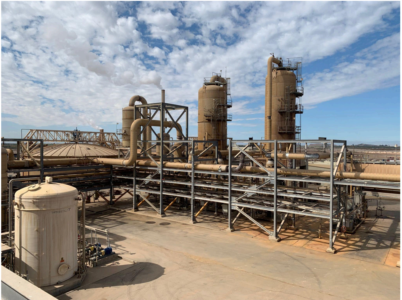
The John L. Featherstone (Hudson Ranch I) Geothermal Power Plant, operated by Cirq, where EnergySource Minerals is developing lithium. Photo by James Blair.
